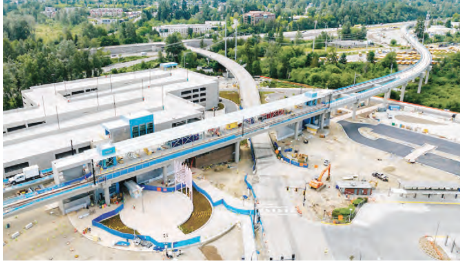
Aerial picture of Lynnwood Link Transit Station progress as of January 2024. SOURCE: Sound Transit.
