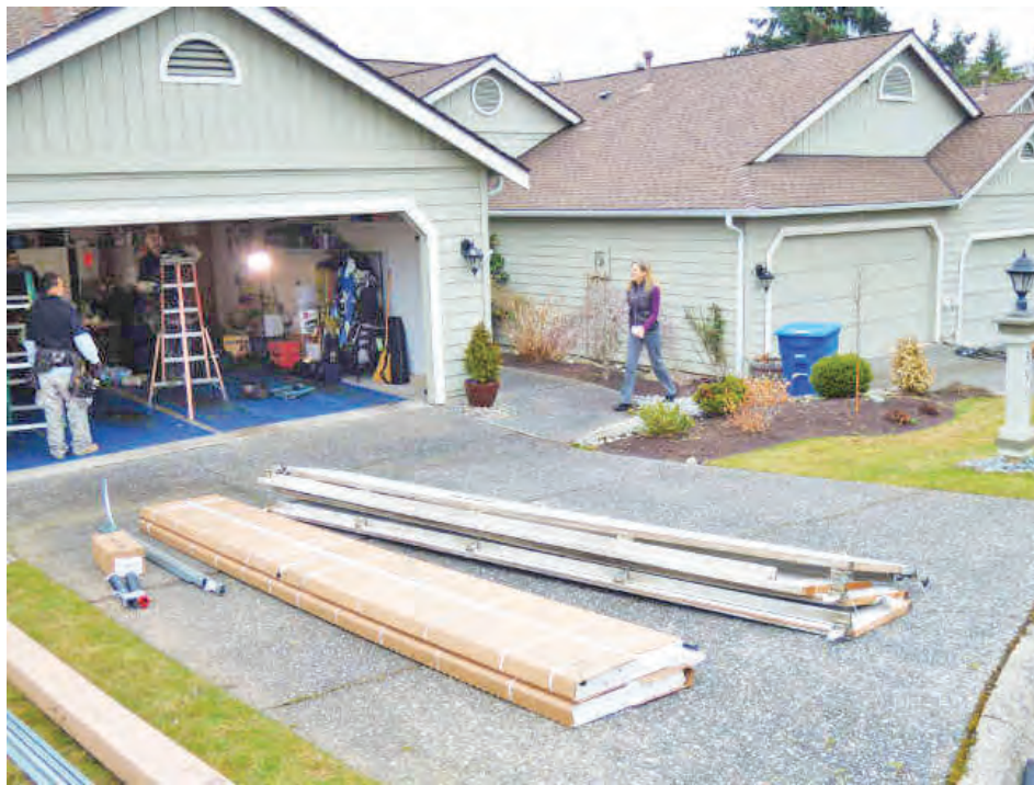
The Elite team repairing a garage door. SOURCE: Elite Garage Door and Gate Repair.
