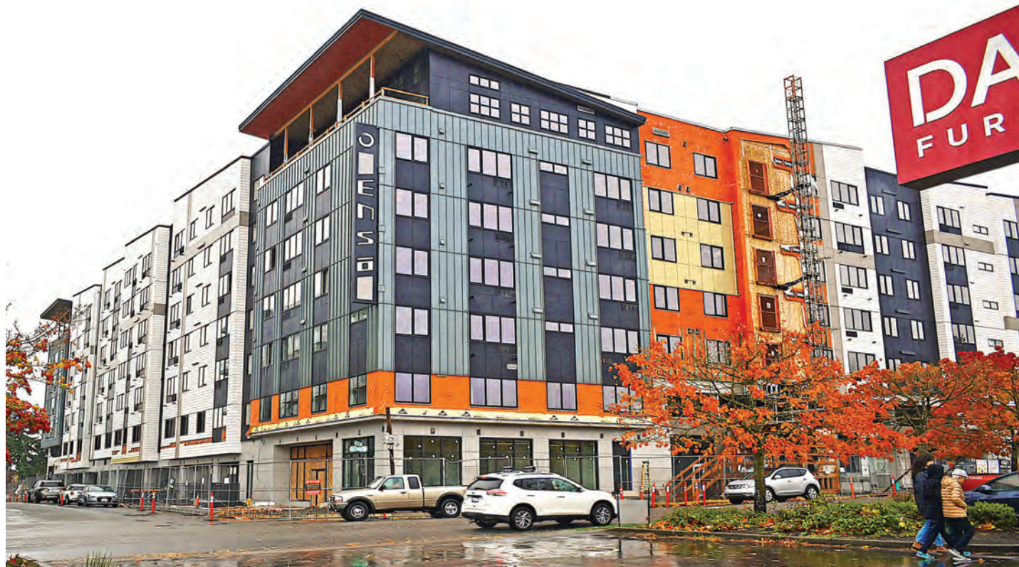
ENSO, a mixed-use development being constructed in Lynnwood's City Center. Lynnwood Times | Mario Lotmore
